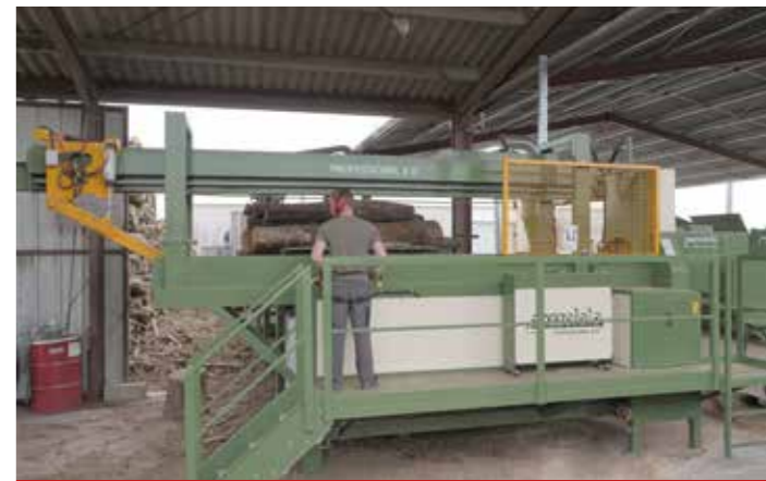
Platform for control board with stairs
